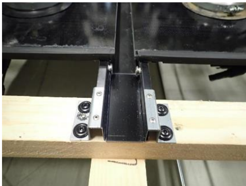
Fig. 2: details of installed system prior to start testing
